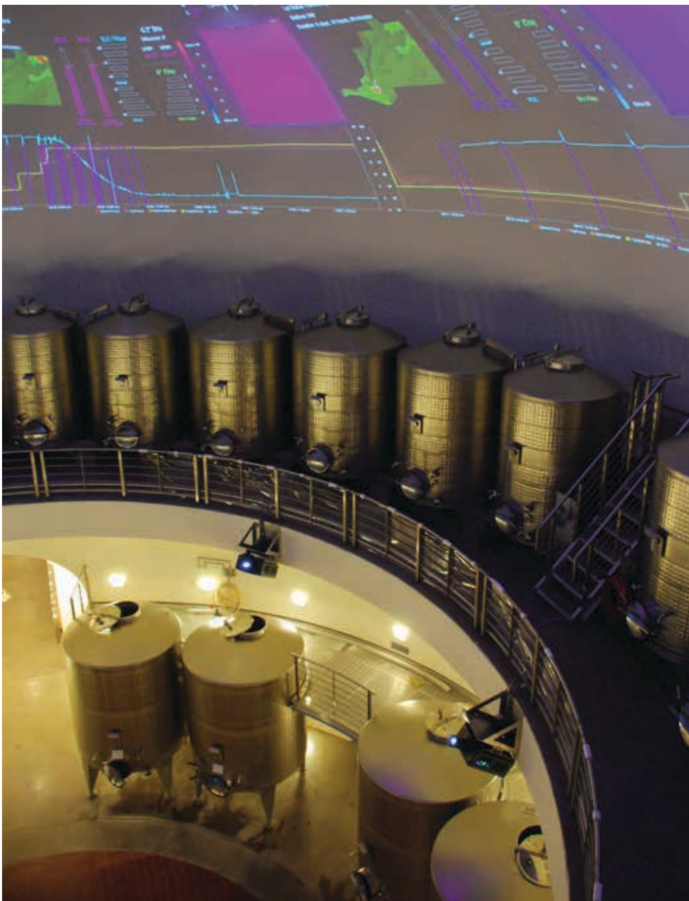
An Acrolon PM-4000 controller at each tank provides local control and link to TankNET web-server for projected visualizations, remote management and advanced data-mining by FELICS.
