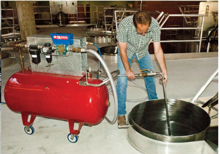
Mobile Pulsair Tank Mixer on mezzanine level. Winemaker positions the wand through the cap to the tank bottom, injects pulses of filtered compressed air under the cap, and moves the wand to different places under the cap until the must is well-mixed.
