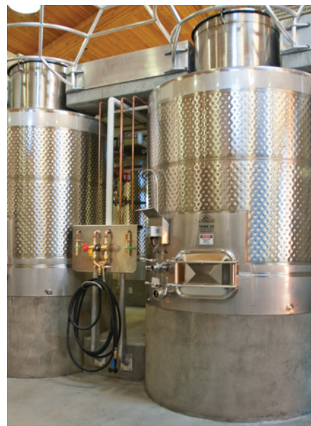
Tanks on concrete pedestals, with access to hot water, cold water, nitrogen, and compressed air. The tanks are “skirted” — welded to cover the gap between the bottom of the tank and concrete, so no water can get underneath the tank when cleaning or spraying down the outside.
